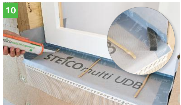
Application of STEICOmulti fill adhesive beads e \leq 30 cm for the elastic fixing of the windowsill. Tip: Compriband strips glued at an angle guide any moisture that may enter safely to the drip edge.
